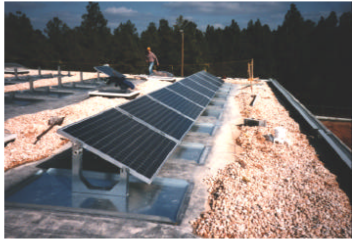
Installation of a ballasted roof mounted PV system for peak shaving at a textiles manufacturing plant.
